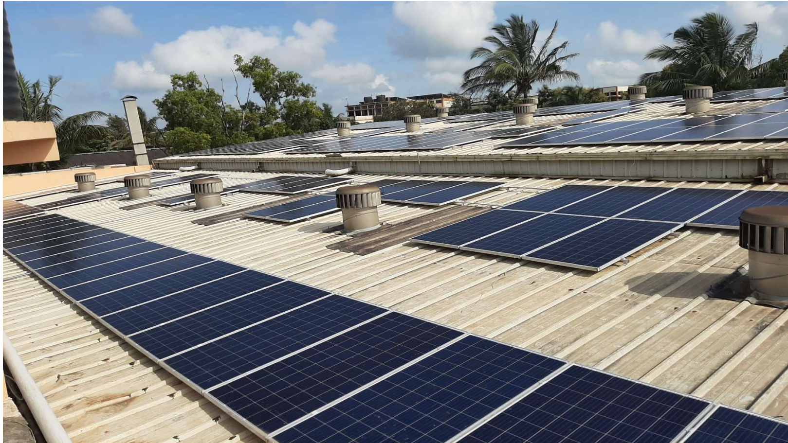
Captive Power Generation through Roof Top Solar Plant
